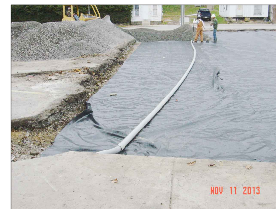
Fiber Optic Conduit under Parking Area
